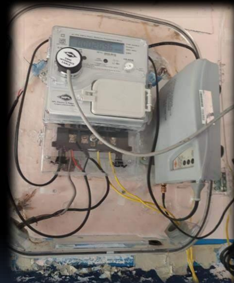
Installed meter with wires inplace
